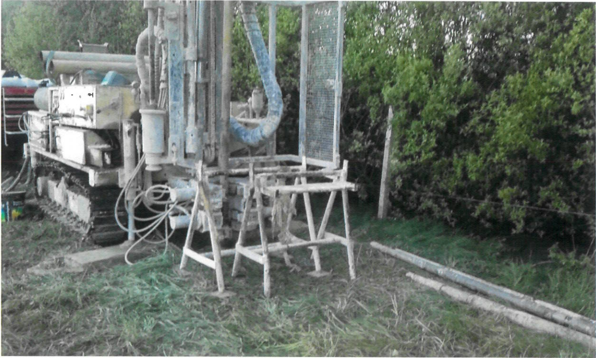
Figure 7: RC 10-09 being carried out on the 26 th April 2017 showing pollution to a tributary of the Lismakeery Stream
